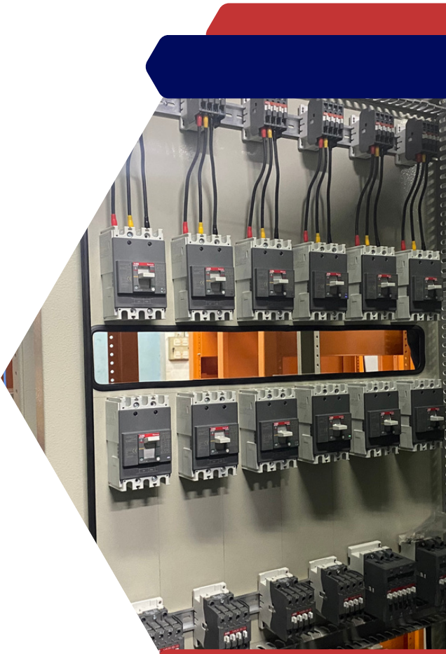
600 Kvar Capacitor Bank Panel
