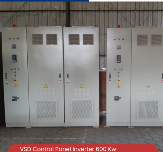
VSD Control Panel Inverter 600 Kw SPAM Project, Bali
