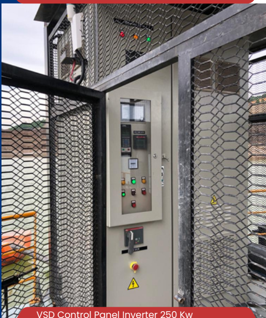
VSD Control Panel Inverter 250 Kw Project Bukit Asam
