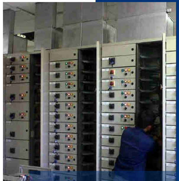
Motor Control Center Panel Merak Energy Project
