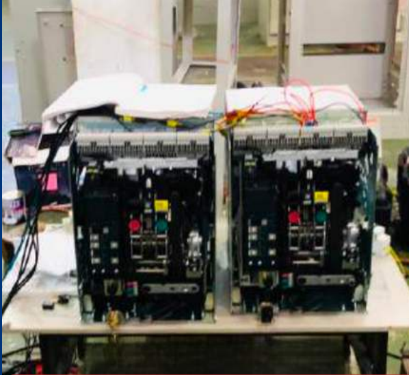
Retrofit Air Circuit Breaker Switchgear MCC 6A SS#2001K Utilities Plaju
