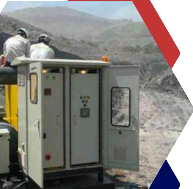
Dewatering System 110 Kw Inverter Panel Freeport Timika
