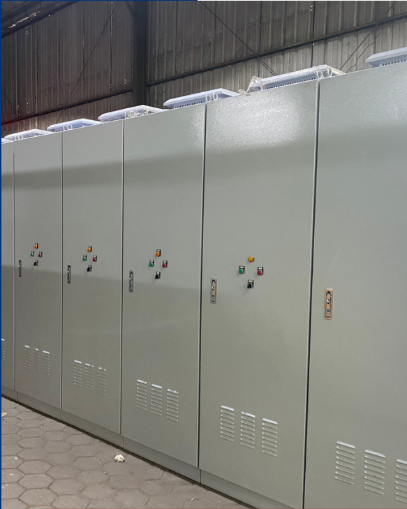
PLC Based Pump Control Panel For Supporting Water Treatment Plant at Medan Johor
