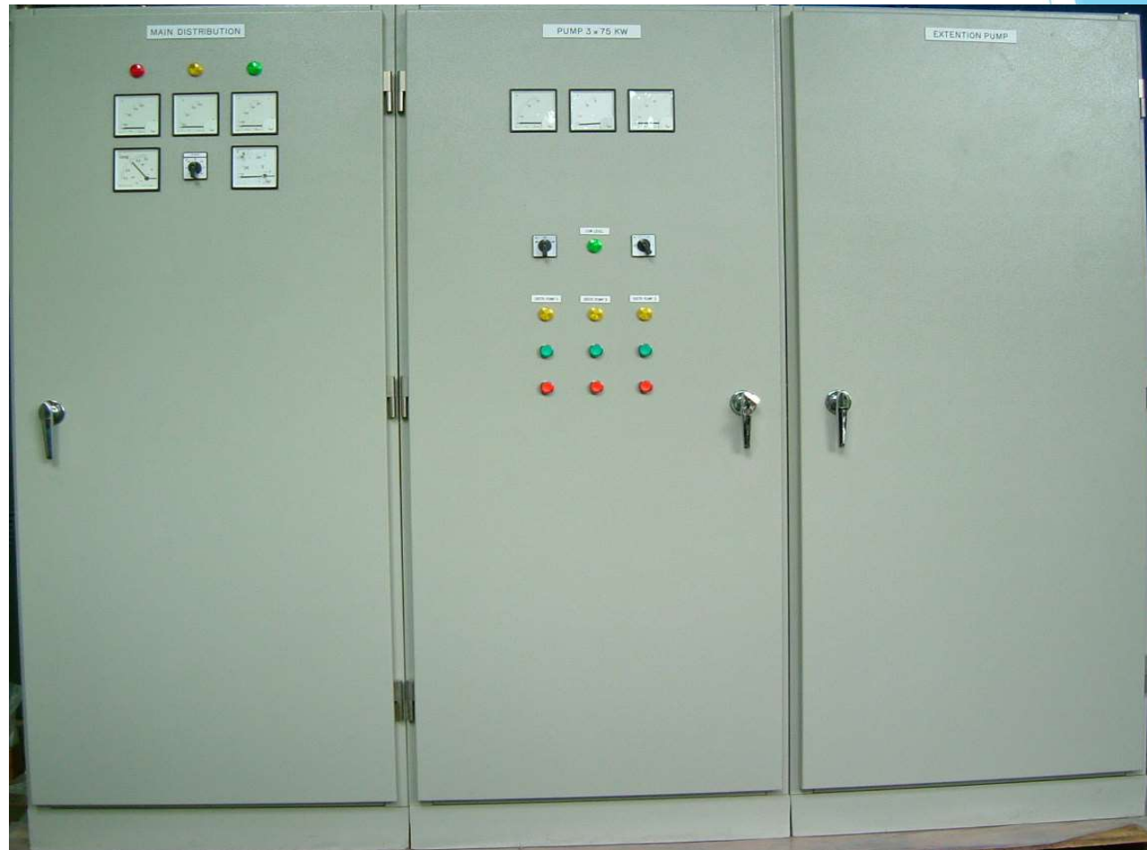
FRONT VIEW INCOMING, PUMP PANEL & EXTENSION PANEL
